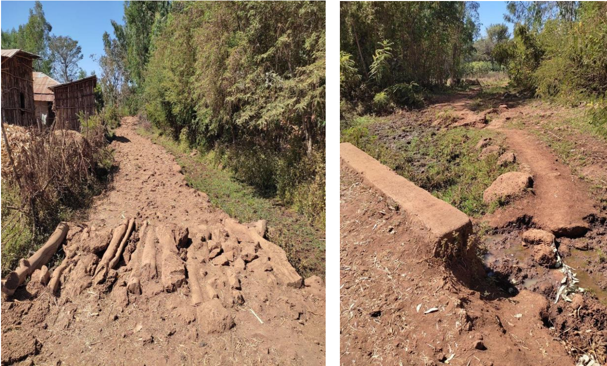
Figure A-2: Poorly planned and constructed foot trail, failing due to lack of a cross drainage structure
